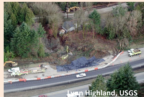
Highway 101 landslide after the 2001 Nisqually earthquake
